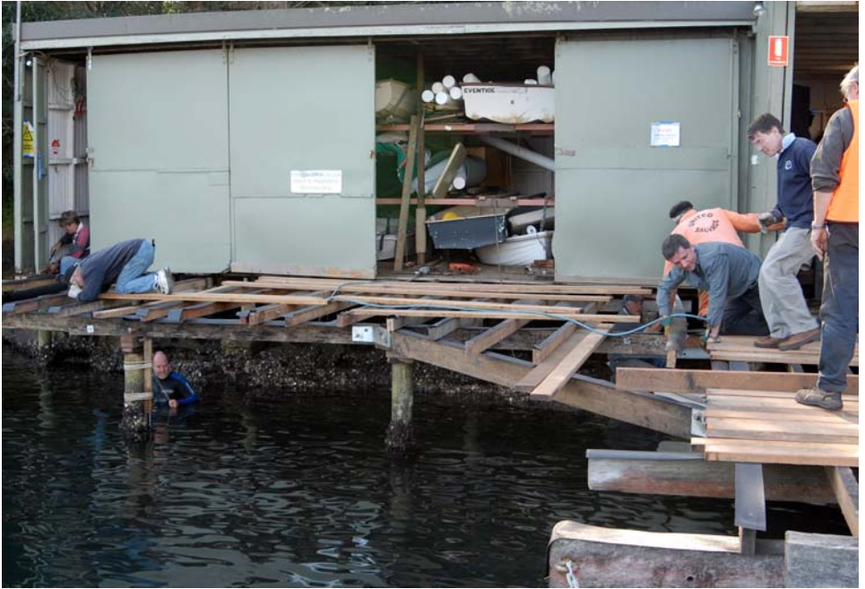
The new deck taking shape, but Bruce Dover is still in the water
