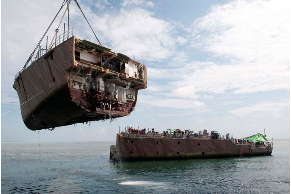
The bow section of Guardian being lifted clear of the reef on 26 March by the crane barge Jacson 25
