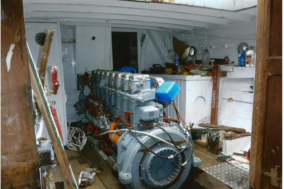
Martindale's engine room with the restored engine
