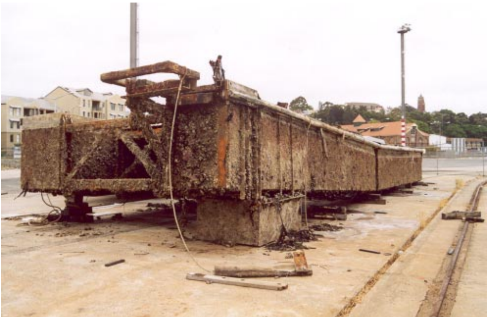
11 November — The old pontoon on the wharf at No. 2 White Bay awaiting demolition. Most of the material was sent to the tip (below)
