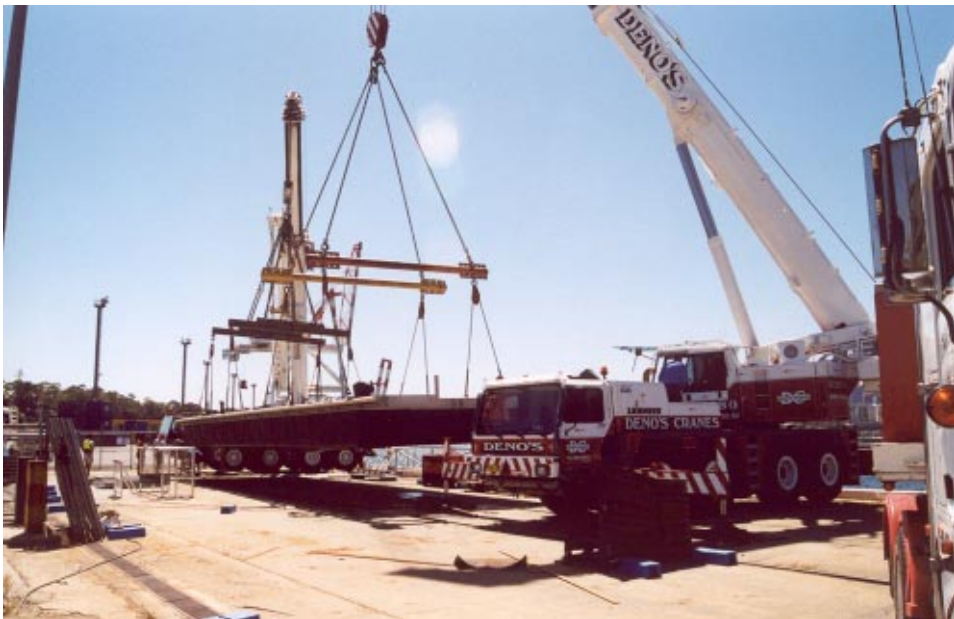
7 November — Launching day. After lifting, welding of the HDPE was completed. As it happened, one of the cranes proved to be not up to the job, and the pontoon was put down again to await the help of another, 120 t, crane (above)
