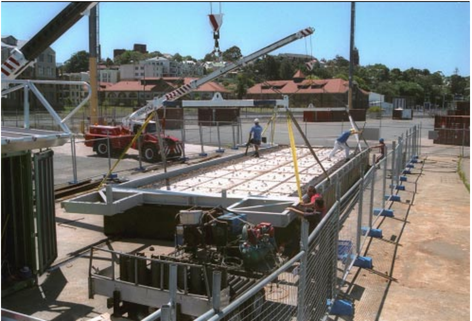
14 October — The concrete deck is surrounded by a steel frame, seen here being lowered into position. It was galvanised and painted with a marine epoxy paint scheme after fabrication. It is made so it can be removed in sections if repairs are ever need in future (above)
