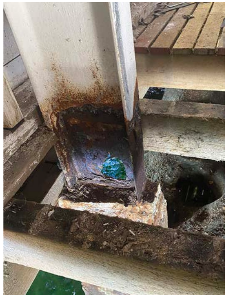
The need for the work was obvious when the column was exposed
