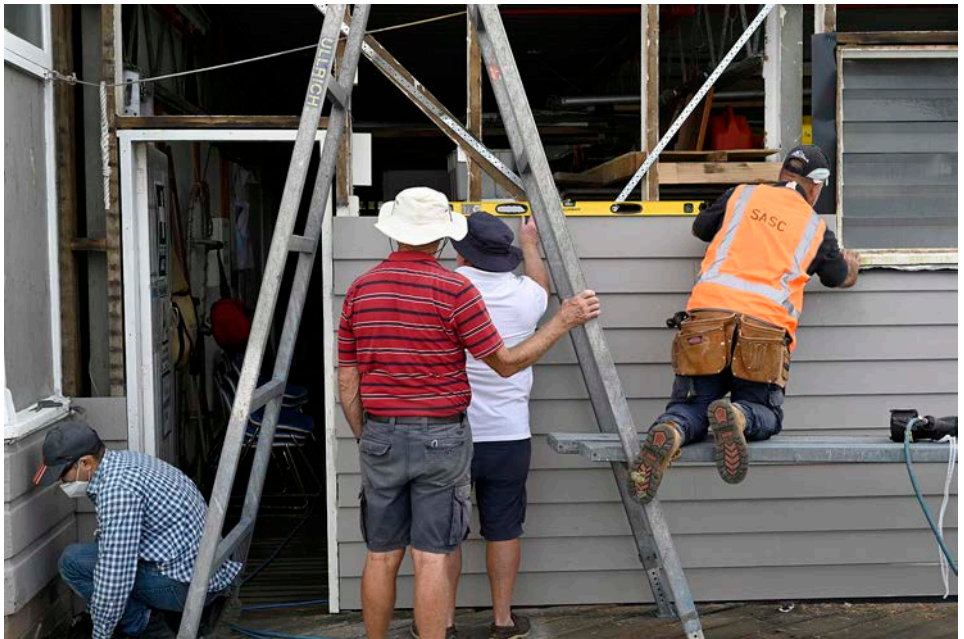
Keeping everything level on 8 May as the boatshed gets a new wall
