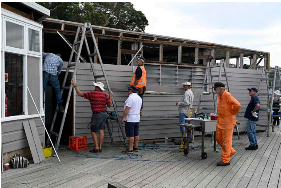
Trevor Cosh (in the orange overalls) keeping an eye on the workers
