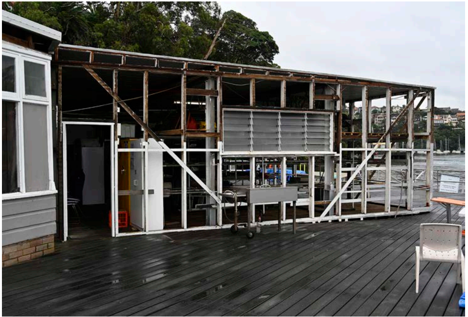
The boatshed on 5 May after all the asbestos-related material had been removed
